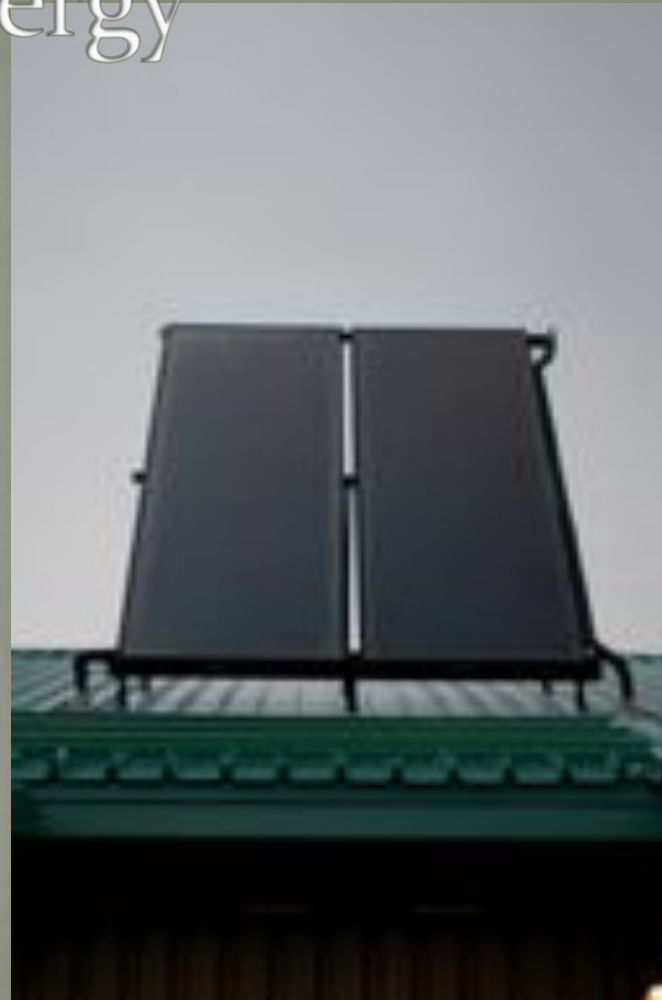
Solar thermal panels in Nenana
