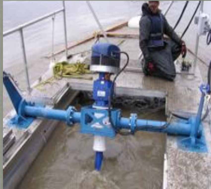
Prototype in-stream turbine installed in Yukon River.
