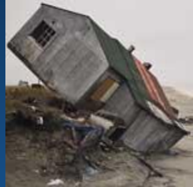
Shishmaref house undermined by coastal erosion
